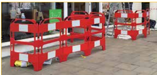
Adhering to the road code contemplated in the DPR 12/16/1992 n.495 and subsequent modifications.
